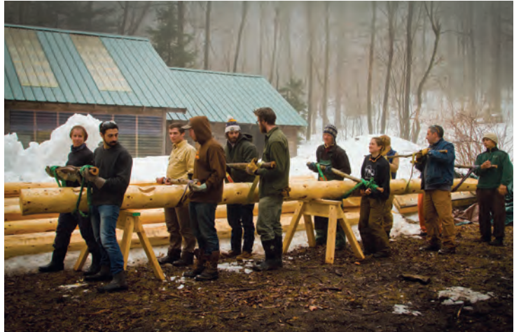
Staff and crew carry a rafter to create the spiraling roof frame of the round house at Flying Cloud in winter 2014.
